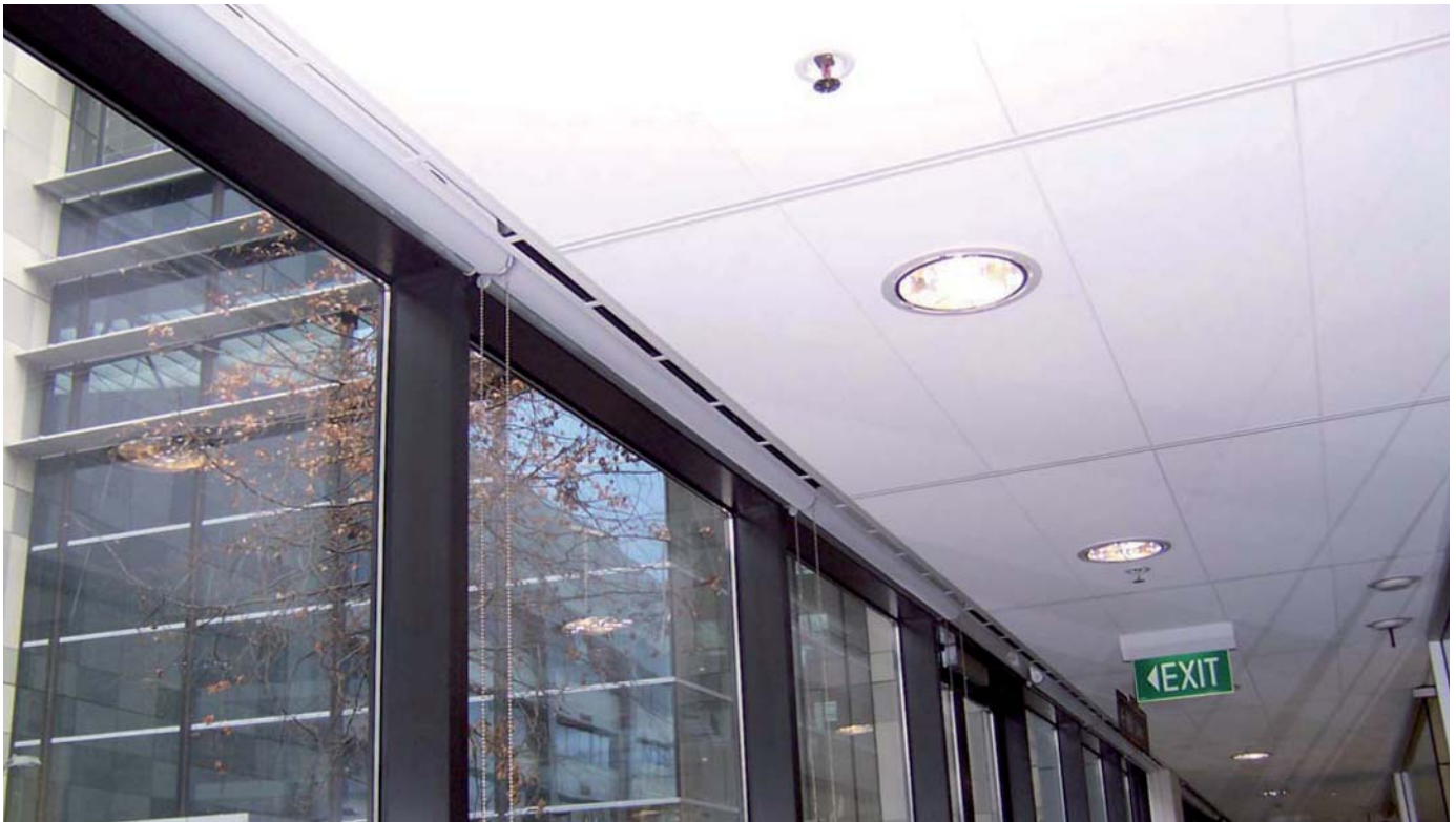
3-Sided Pelmet with slotted Air Diffuser Face Plate – Modular Grid and Ultima panel – Woolworths HQ, Sydney
